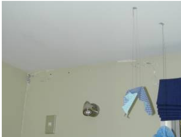
Plate 4 Fracture of Plasterboard along a Line of Fasteners
