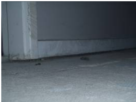
(a) Element Uplift After Earthquake
