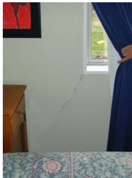
(b) Diagonal Crack at Corner of Window
