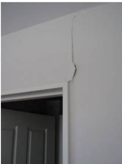
(a) Crack of Joint above Door
