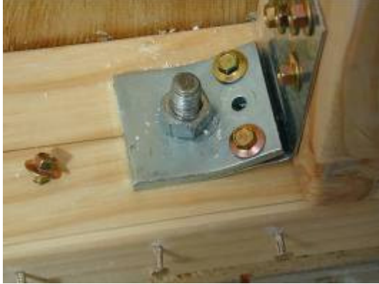
(a) Damage to Hold-Down
