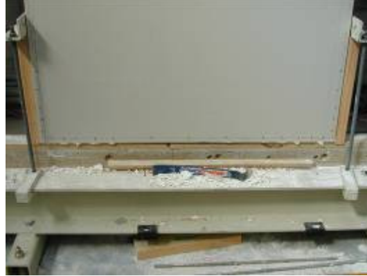
(b) Damage to Bottom of Sheet
