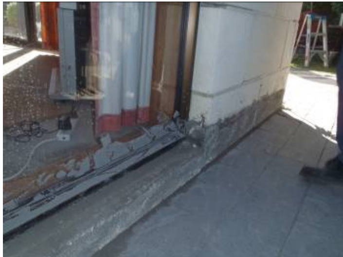
Plate 12 Liquefaction around a Brick Cavity House
