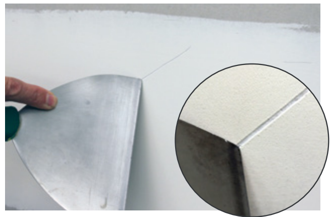
FIGURE 4: A scratch in a basecoat not properly set goes deep/right through and indicates is it soft.
