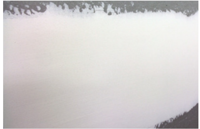
FIGURE 2: Basecoat compound is lighter in colour and shows it has not set properly.
