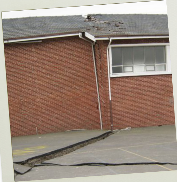
School hall broken in half due to subsidence
